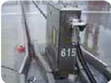
Yard Junction Box with circuit breaker protection, providing the interface to connect the cable reel to the yard power supply
